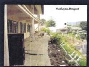
e) Doors jamming, walls tilting, floors cracking
