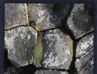
d) presence of open fractures
